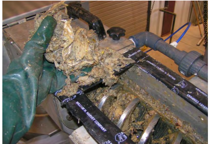
Removing Items Caught in Treatment Plant Auger
