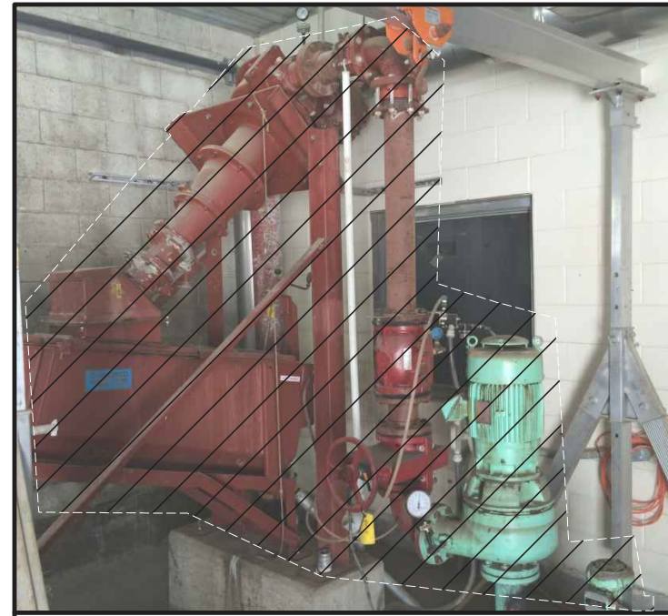
PHOTO 3 ③ DEMO GRIT REMOVAL SYSTEM INCLUDING GRIT CLASSIFIER, GRIT HYDRO CYCLONE, GRIT PUMP, CONCRETE OVER BASIN, & GRIT EQUIPMENT IN BASIN AS NEEDED TO INSTALL NEW GRIT SYSTEM.
