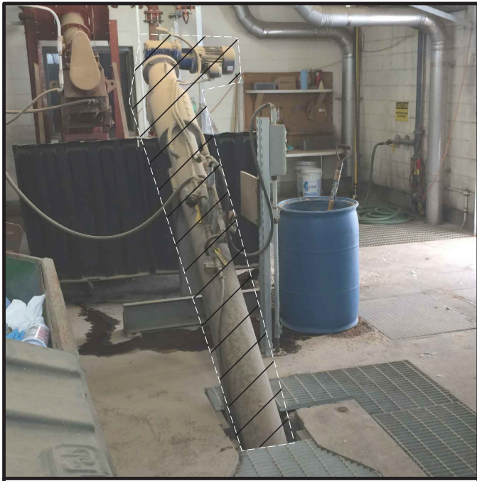
PHOTO 1 ① DEMO EXISTING MECHANICAL SCREEN. SALVAGE ELECTRICAL & CONTROL PANEL TO BE REUSED WITH NEW SCREEN.
