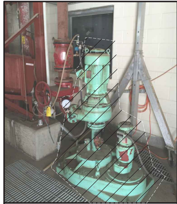
PHOTO 2 ② DEMO EXISTING GRIT SYSTEM INCLUDING DRIVE, GEARBOX, PUMP, GROUT FILLET, IN SUMP PIPING, EQUIPMENT IN BASIN, AND GRIT CLASSIFIER.
